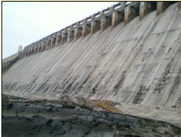
Figure 1B: Cavitation damage on spillway profile of Nagarjunasagar Dam.
