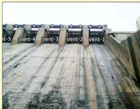
Figure 1A: Cavitation damage on spillway profile of Nagarjunasagar Dam.
